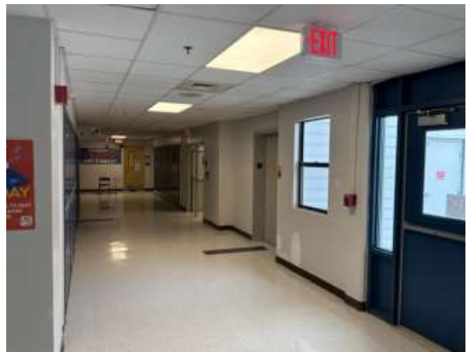
48 - FIRE ALARM SYSTEM DEVICES
