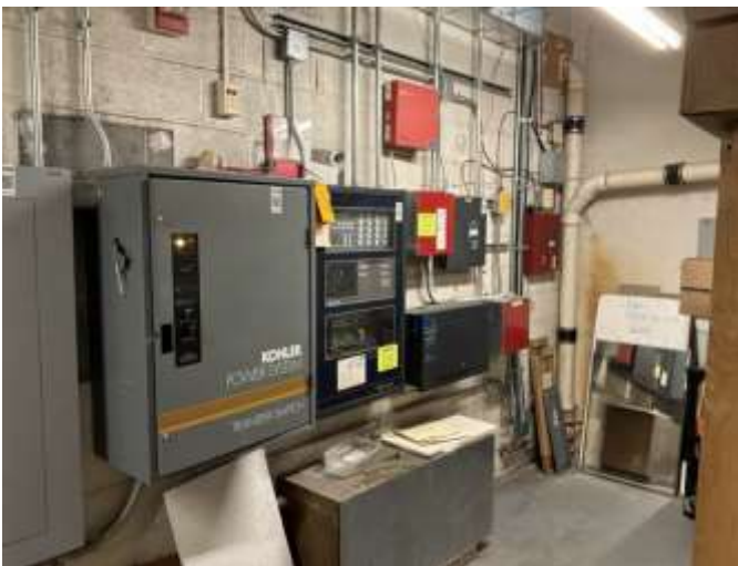
47 - FIRE ALARM CONTROL PANEL
