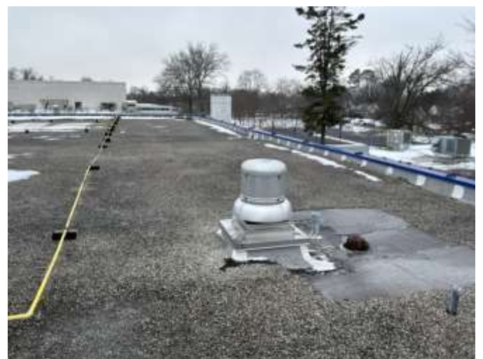
42 - TYPICAL EXHAUST FAN
