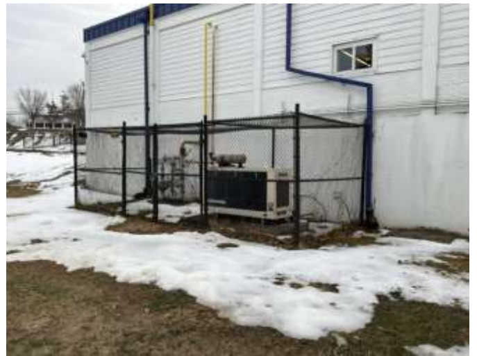
46 - EMERGENCY POWER GENERATOR
