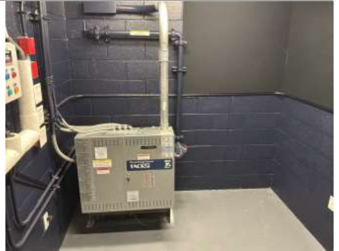
32 - ELEVATOR MACHINE ROOM
