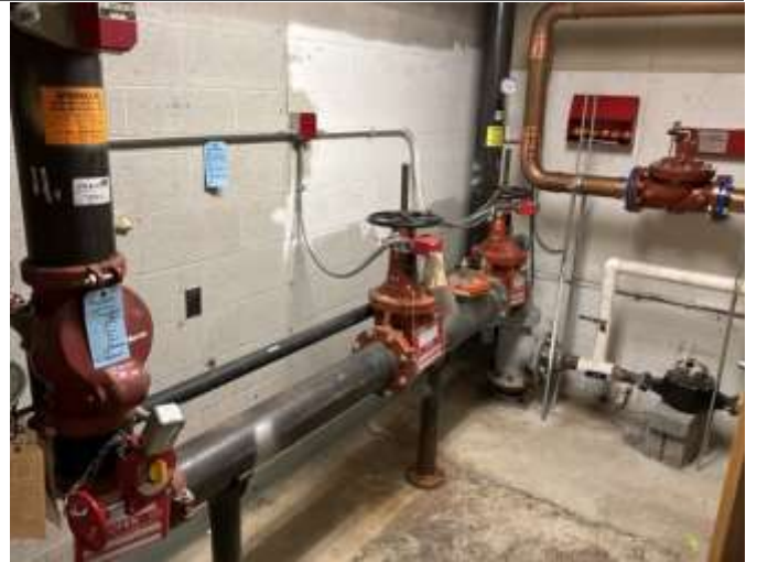
44 - FIRE BACKFLOW PREVENTER
