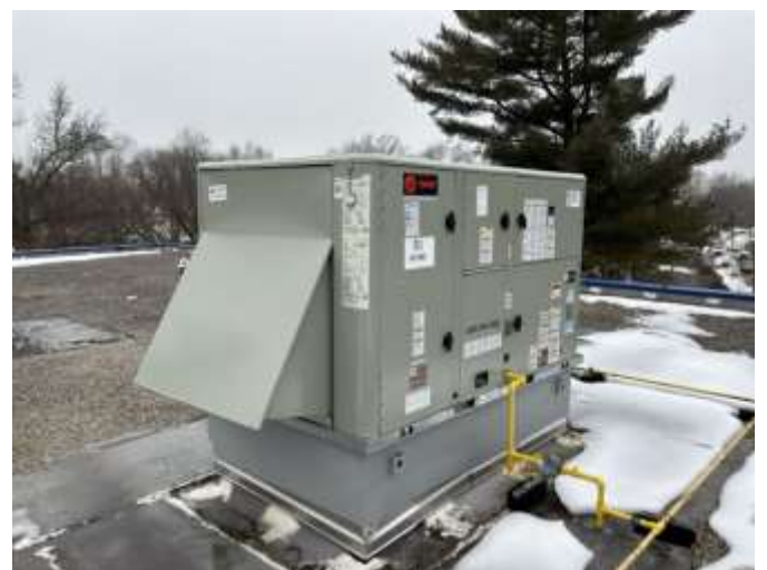
36 - TYPICAL PACKAGED UNIT
