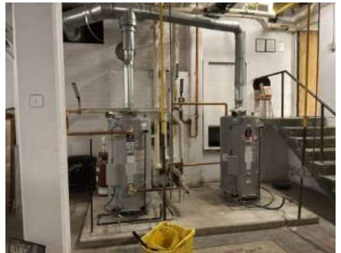
34 - DOMESTIC HOT WATER SUPPLY
